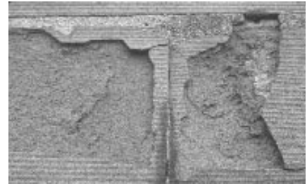
Contour scaling (top) and disaggregation (bottom) are two commonly found forms of brownstone deterioration.
