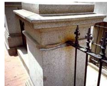
The iron stain on this granite post may be removed by applying a commercial rust-removal product in a poultice. Photo: NPS files
