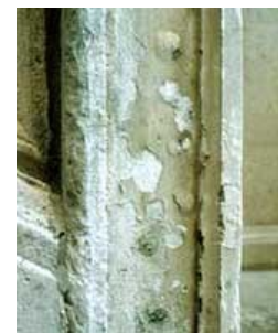
This clear coating has failed and is pulling off pieces of the stone as it peels. Photo: NPS files
