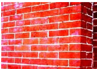
Improper cleaning methods may have been responsible for the formation of efflorescence on this brick. Photo: NPS files.
