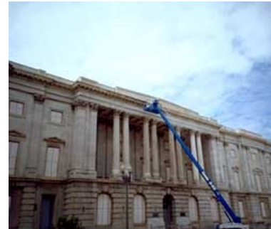
Low-to-medium-pressure steam (hot-pressurized water washing) is a gentle method of softening heavy soiling deposits and cleaning historic marble. Photo: NPS files.
