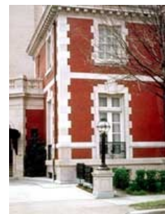
The decorative trim on this brick building is architectural terra-cotta intended to simulate the limestone foundation. Photo: NPS files.
