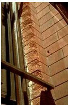
Brick molding next to the window has been severely abraded by sandblasting to remove paint. Photo: NPS files.
